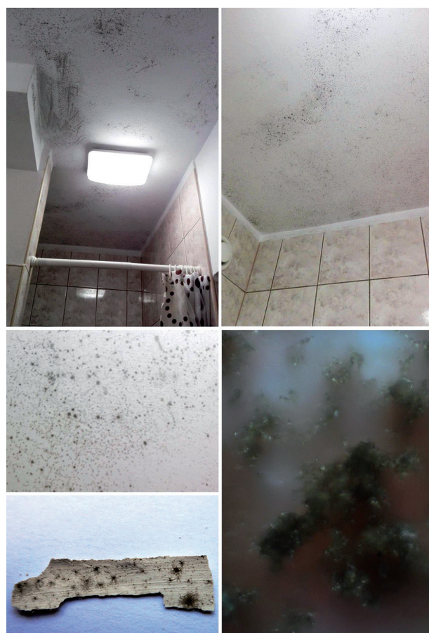
Fig. 1. The dark stains covering bathroom ceiling in the studied facility – the samples were collected from the paint scrapings.
